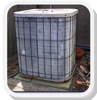
PICTURE OF AN AIR CONDITIONING CONDENSER.
